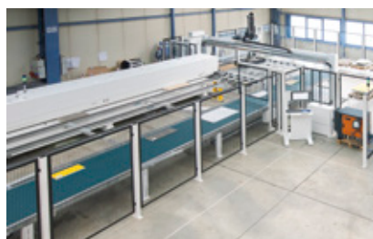
Equipment to achieve CE-conformity: protection grid along the complete return section
